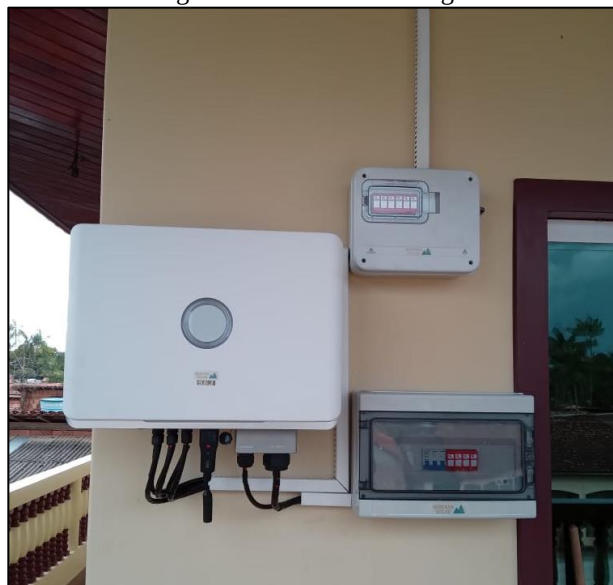
Figura 15 - Inversor e strings box.
